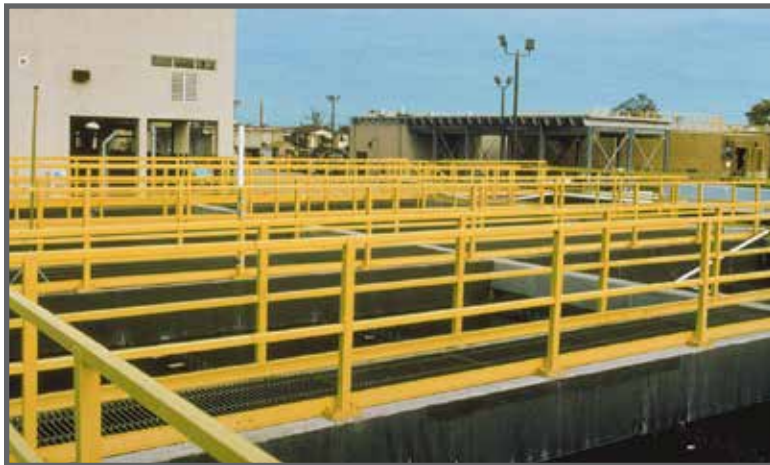
Square tube railing manufactured with Dynaform component products offer long life in the corrosive environment of this wastewater treatment plant.
