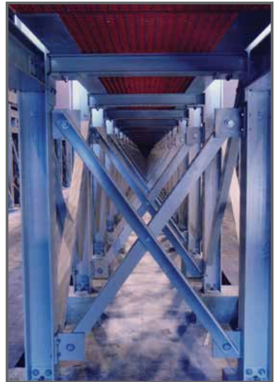
As the chosen product for a highly corrosive battery manufacturing facility, this Dynaform platform will provide years of service.
