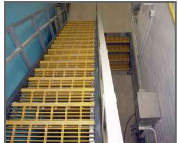
The stairway above utilizes Fibertred moulded stair treads to provide tank access at a pumping station.
